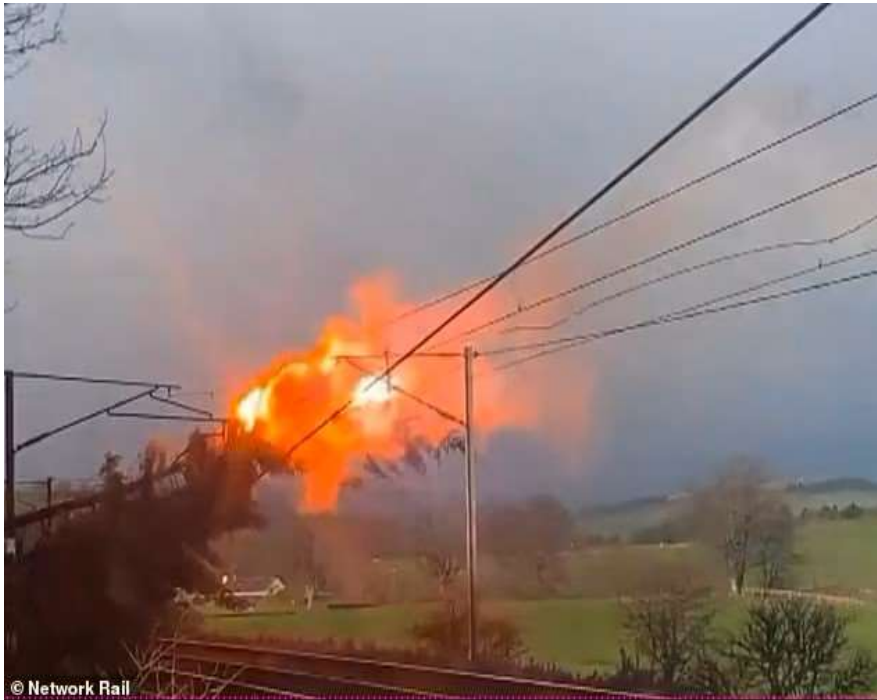
Fig – 5 – A fire on Overhead cables between Motherwell and Lockerbie Scotland after a Stormy Weather
